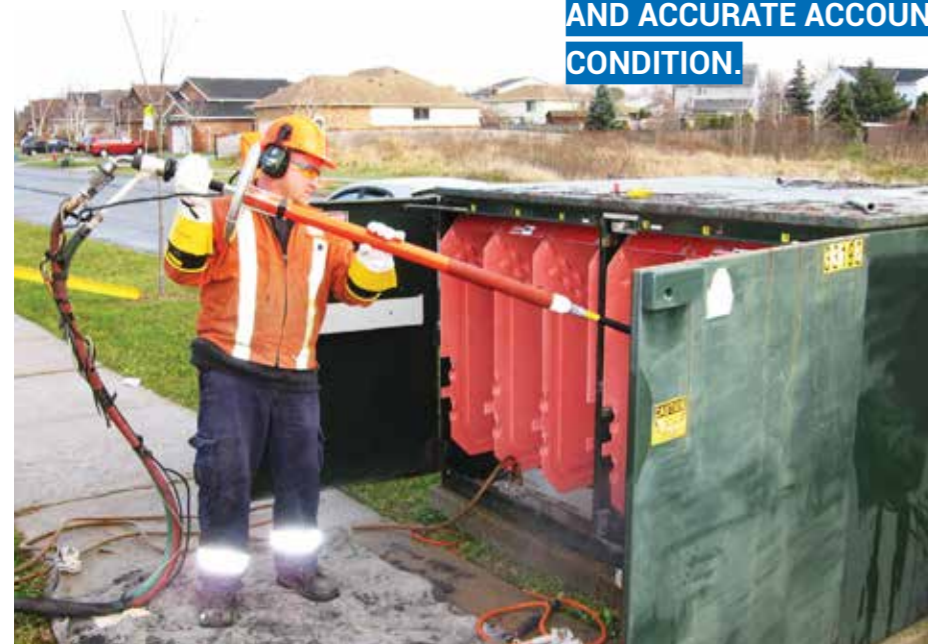
Figure 1. An electrical service technician applies simple dry ice cleaning on a residential transformer.
