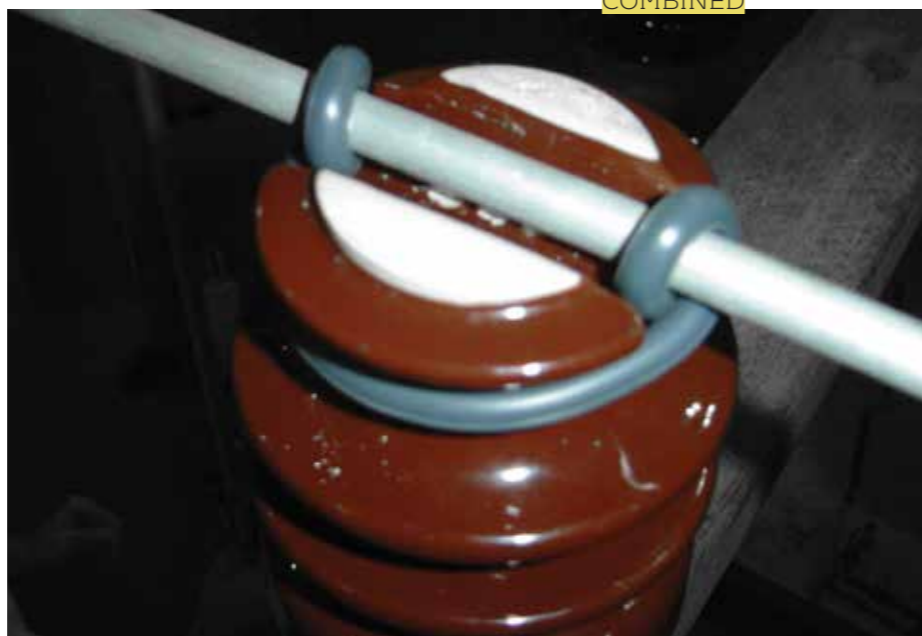
Figure 2. Tracking has begun to erode the enamel coating on this insulator. Moisture can impregnate and either super heat (arcing) or freeze. The insulative properties are failing and partial discharge will only worsen from here.
