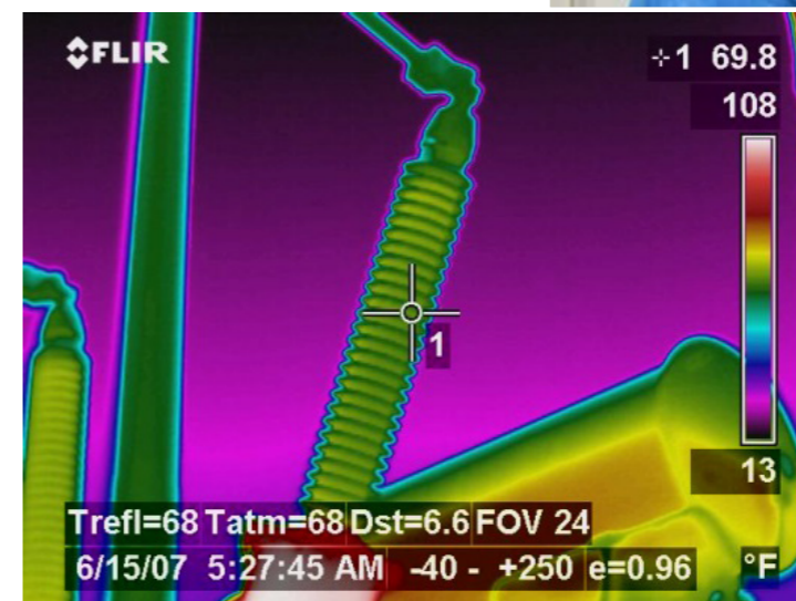
Figure 3. Infrared did not discover any electrical anomalies; however, additional ultrasound scans revealed the onset of early stages of corona discharge.
